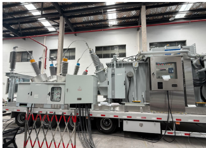
Guatemala | TRELEC 69 kV Mobile Substation Project
