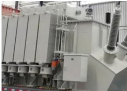
Italy | 69kV Trailer-Mounted Substation
