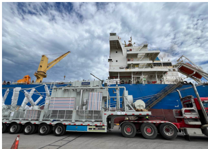
Honduras | 132kV Mobile Substation
